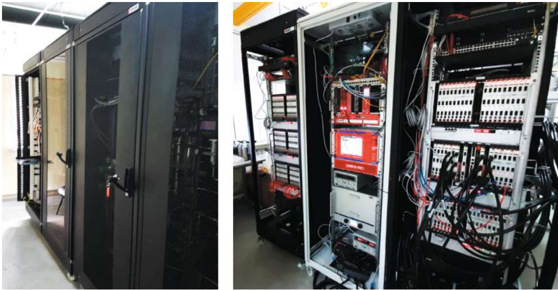
Fig. 6. Racks with gas system for setup and data acquisition system.
