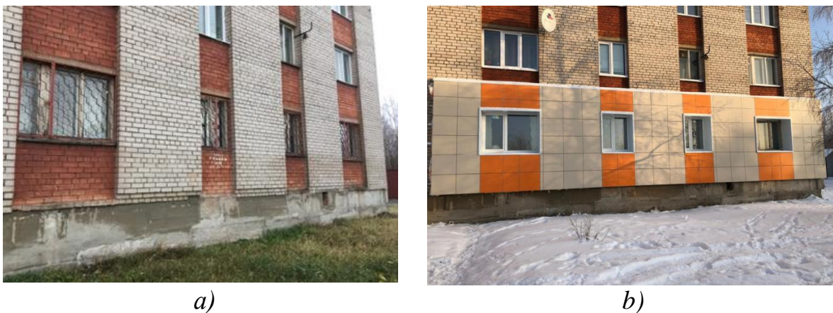
Picture 1. Facade of the NArFU dormitory: a) before repair work; b) after repair work.
