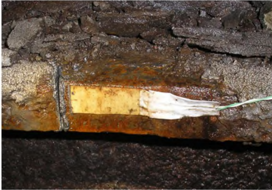
Fig. 4: Photo of a pig-iron wall of a trunk with the strain gage after application of a method of partial unloading
