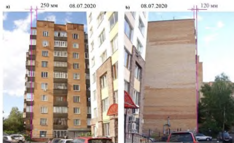
Figure 2: The size of the tilt: a) a residential building on Zelenko street (Kursk); b) a residential building on Mirnaya street (Kursk)
